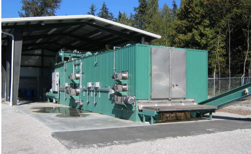
UBC's In-Vessel Unit
