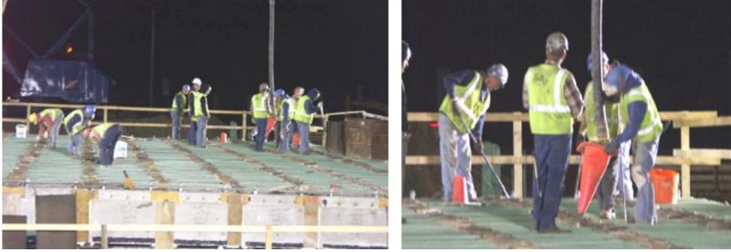
Figure 2-6. Grouting adjacent box-beam shear keys using type R-2 grout (Oakland Drive over I-94, MI)
