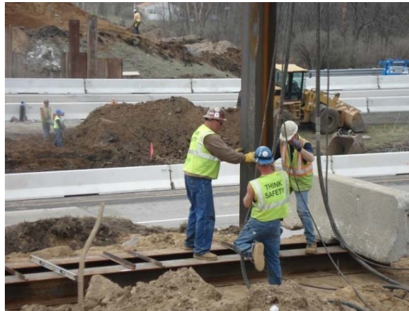
Figure 5-16. Template used for maintaining pile driving tolerances (Source: Photo courtesy of MDOT)
