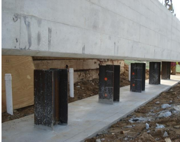
Figure 5-17. Concrete slab on ground to maintain the proper grade for placing the abutment stem (Source: Photo courtesy of MDOT)
