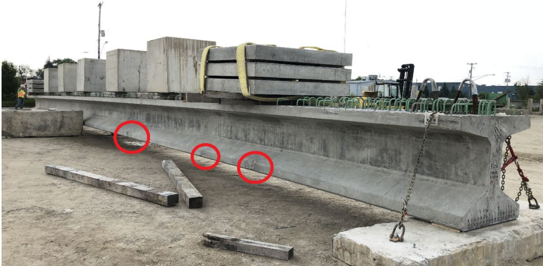
(a) A girder with major nonconformance
