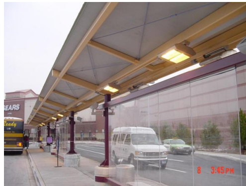
Figure 5-28. Infrared heaters implemented at a bus stop (Source: MEHA 2015a)
