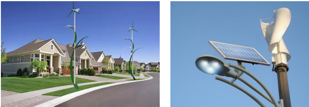
Figure 5-6. Wind-solar hybrid street lighting systems (Source: Sunning 2015)
