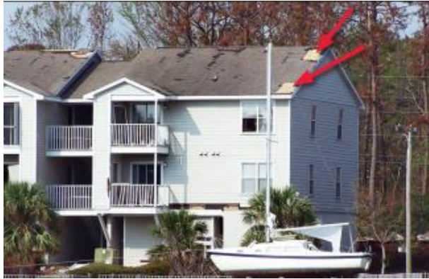
(a) Roof covering damage
