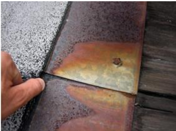
Figure 3-37. Rusting of metal flashing and fasteners (Kelly Roofing 2018)
