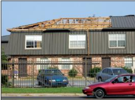
Figure 6. Blow-off of nailers caused these panels to progressively fall. The nailers were installed directly over the trusses. In an assembly such as this where there is no decking, there is no opportunity to incorporate an underlayment. With loss of the panels, rainwater was free to enter the building.
