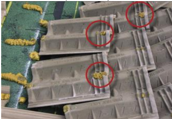
(c) Loss of clay tiles during Hurricane Charley, 2004 (FEMA 2005)
