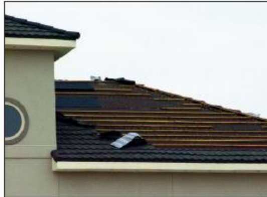
Figure 7. This residence had metal shingles that simulated the appearance of tile. The shingles typically blow off the battens, but some of the battens were also blown away.
