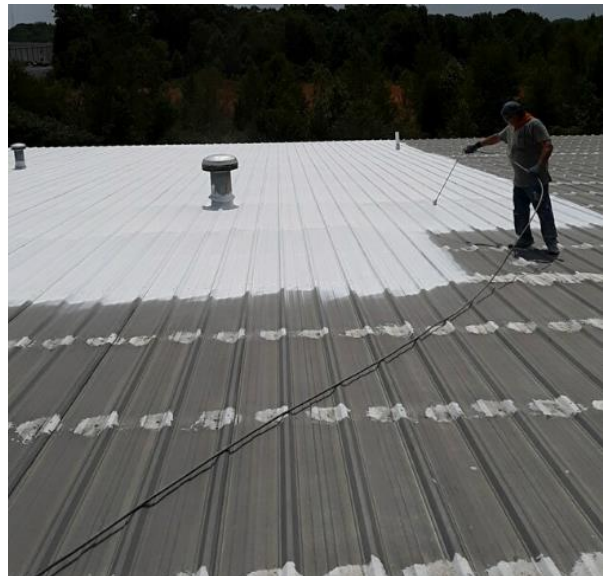
Figure 3-7. Roof coating being sprayed over a metal roof after screw heads are sealed with mastic (Armor Garage 2018)
