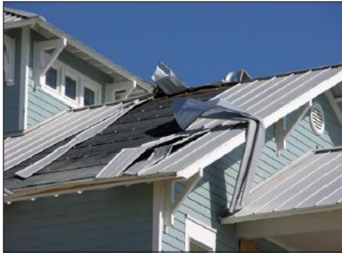
Figure 2. This architectural panel system has concealed clips. The panels unattached from the clips. The first row of clips (just above the red line) was several inches from the end of the panels. The first row of clips should have been closer to the eave.
