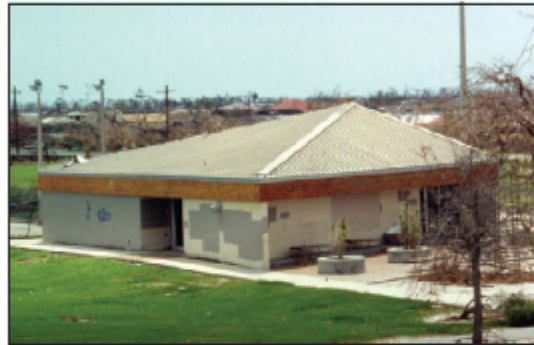
Figure 1. This structural standing seam roof system survived Hurricane Andrew (Florida, 1992), but some hip flashings were blown off. The estimated wind speed was 170 mph (peak gust, at 33 feet for Exposure C).
