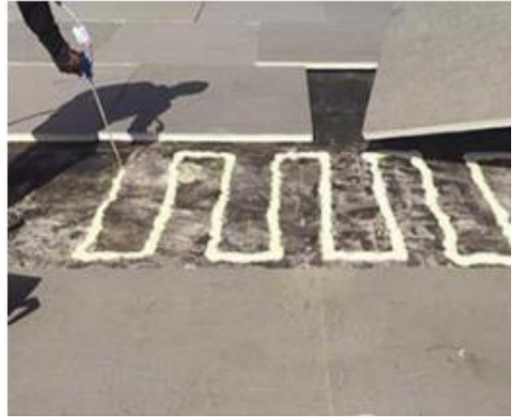
Figure 3-3. Insulation board installation – a spray gun is used for foam adhesive application (ICP Adhesives & Sealants 2018)
