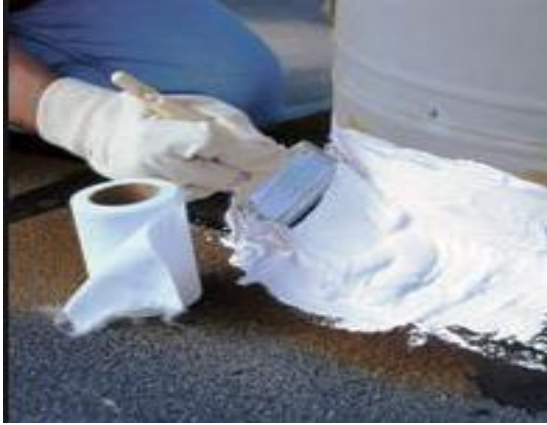
Figure 3-10. Application of a flashing sealant with reinforcing fabrics around a roof penetration using a brush (RoofSource n.d.)
