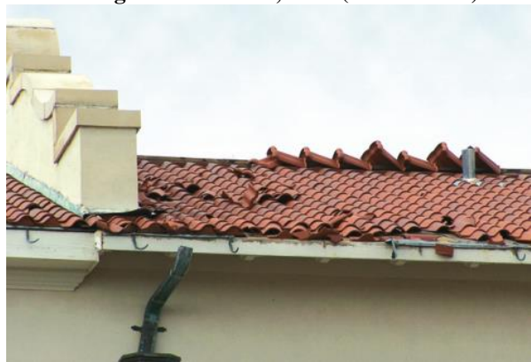
(d) Uplift of ridge tiles during Hurricane Katrina, 2005 (FEMA 2006)
