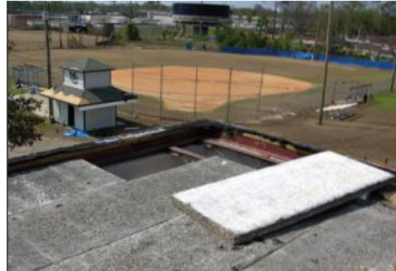
(b) BUR panel blow off at a roof corner
