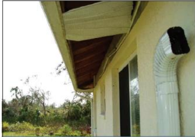
Figure 1. Missing soffit material.
