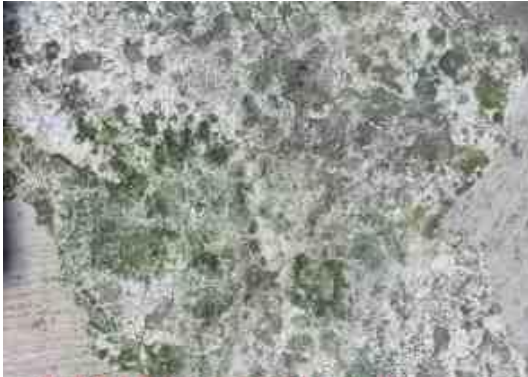
Figure 3-35. Algae growth due to water leakage (InspectAPedia 2015)
