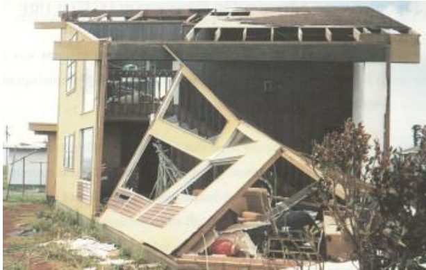
(a) Failure of exterior walls
