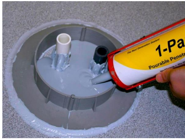
Figure 3-9. Application of a pourable, waterproofing sealer inside a curb surrounding a roof penetration (Conspec materials Inc n.d.)
