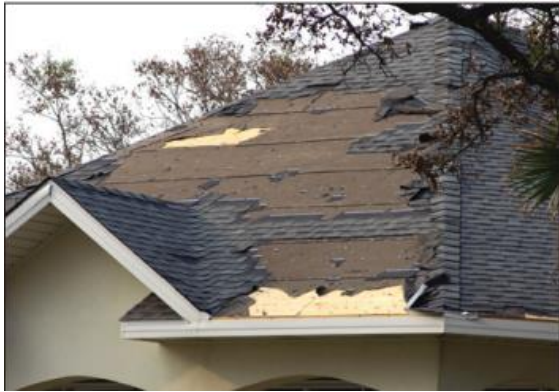
(a) Loss of shingles during Hurricane Katrina, 2005 (FEMA 2006)
