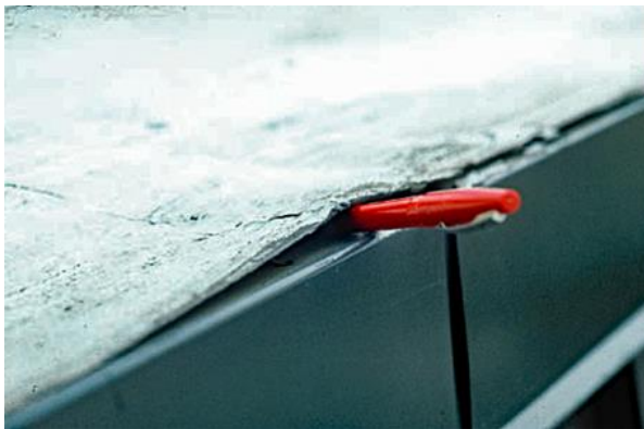
(a) Improper installation of an edge flashing
