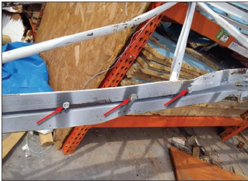
(a) Failed puddle welds that connected the metal roof deck to the top chord of the joist (red arrows) (FEMA 2012)
