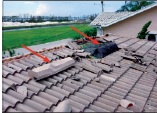
Figure 11. Two off-ridge vents are shown in this photograph. The vent that is covered with roofing felt flipped up and allowed a substantial amount of water to enter the residence. Carpeting, kitchen cabinets, and a large amount of gypsum board had to be replaced because of the water intrusion.
