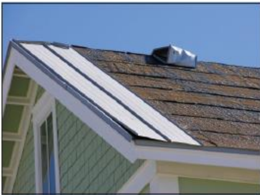
Figure 3. These architectural panel system have snap-lock seams. One side of the seam is attached with a concealed fastener. Although a large number of panels blew away, the underlayment did not.
