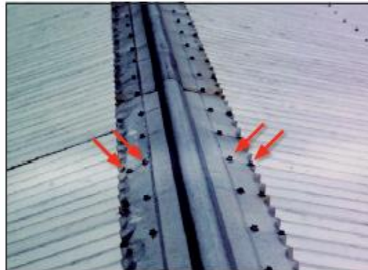
Figure 8. The ridge flashing on these corrugated metal panels had two rows of fasteners on each side of the ridge line.
