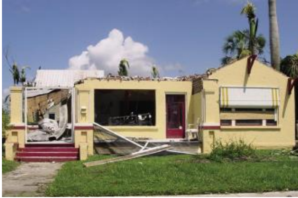
(a) Failure of a wood roof structure in a masonry building (FEMA 2005)
