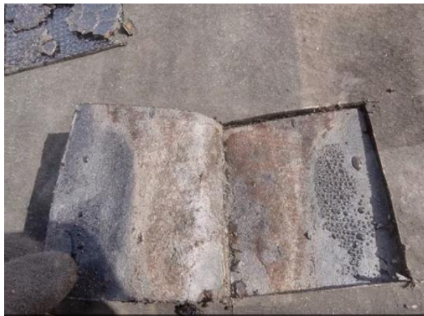
(c) Significant amounts of water between felt layers in BUR
