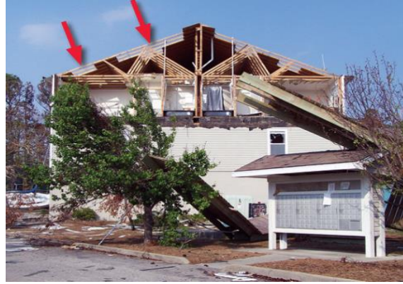
(b) Failure of plywood sheathing in a wood framed building (FEMA 2006)
