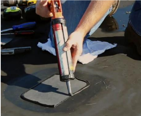
Figure 3-8. Application of a sealant using a caulking gun during an EPDM roof repair (Jurin Roofing Services n.d.)
