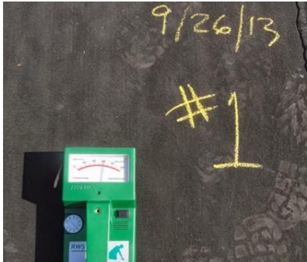
(a) Wet roof reading on electrical capacitance meter
