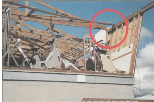
(b) Failure of truss and exterior wall connection
