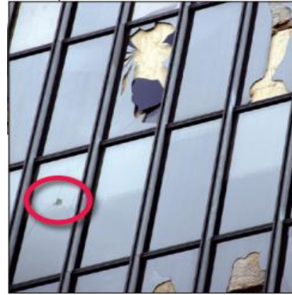
(b) Broken glasses in a façade (FEMA 2006)
