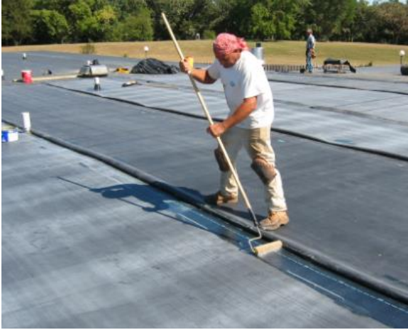
Figure 3-2. EPDM membrane installation – a roller brush is used to apply a liquid adhesive (ERA 2010)
