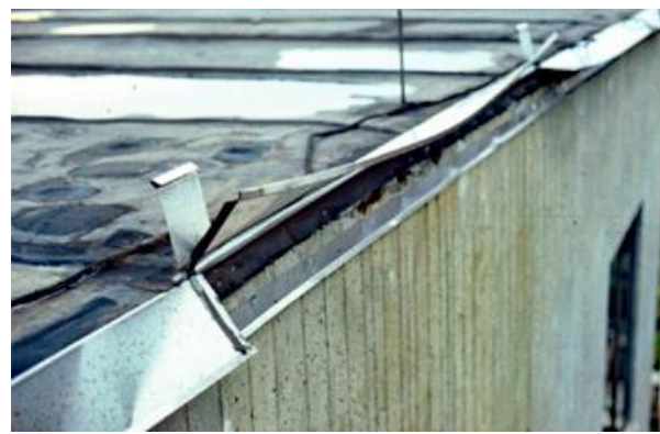
(b) Disengagement of the flashing from the cleat and lift up of the vertical flange
