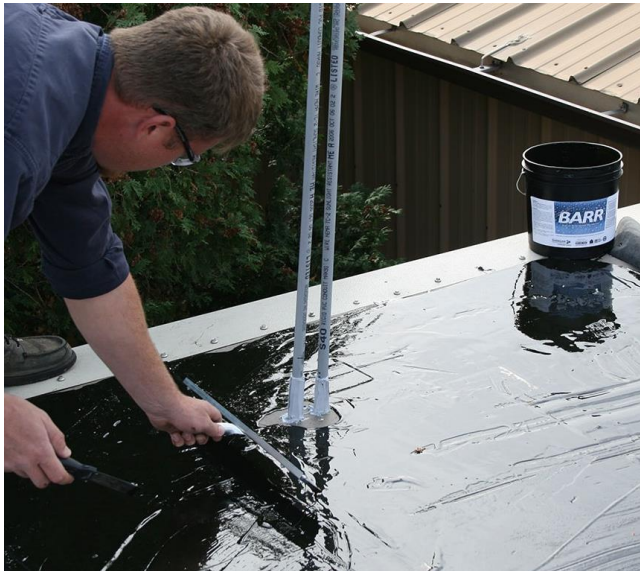
Figure 3-6. A waterproofing coating applied over the membrane using a squeegee (Conspec material Inc. n.d.)
