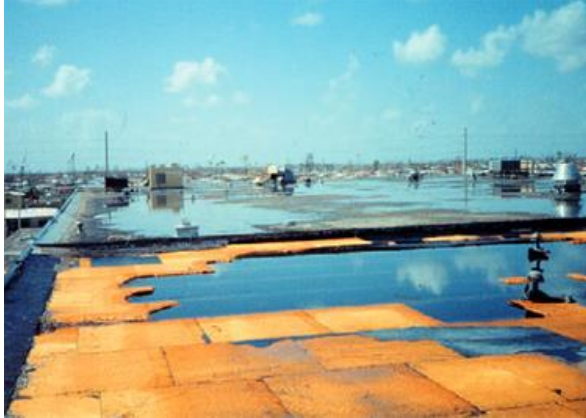
(a) Lifting and peeling off of build-up membrane (Smith 2017)
