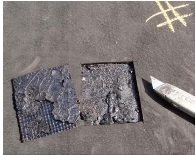
(b) Test cut reveals standing water between membrane and BUR
