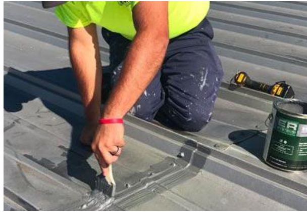
Figure 3-11. Application of a polyurethane sealant at a seam joint of metal roof system using a brush (Jewett Roofing Company, 2016)
