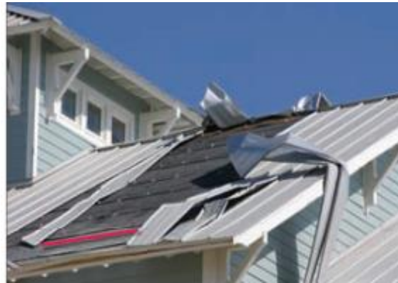
(b) Concealed clips unclipped from the metal panels during Hurricane Ike, 2008 (FEMA 2009)
