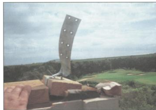
(b) Failure of an undersized and improperly attached metal fastener
