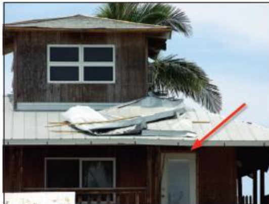
Figure 5. The panels blew off the upper roof and landed on the lower roof of this house. The upper asphalt shingle roof shown had been re-covered with 5V-Crimp panels that were screwed to nailers. The failure was caused by inadequate attachment of the nailers (which had widely-spaced nails) to the sheathing. Note that the hip flashing on the lower roof blew off.
