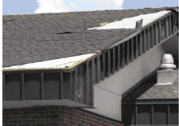
(b) Failure of shingles during Hurricane Charley, 2004 (FEMA 2005)
