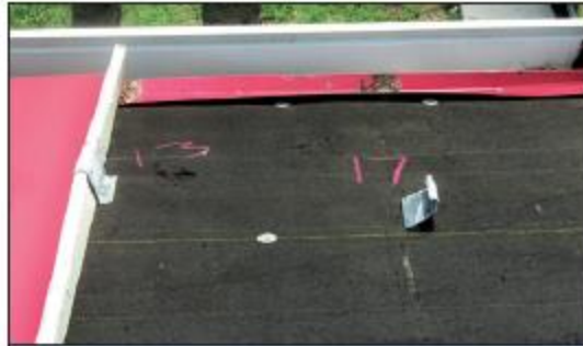
Figure 4. These eave clips were too far from the panel ends. The clip at the left was 13" from the edge of the deck. The other clip was 17" from the edge. It would have been prudent to install double clips along the eave.
