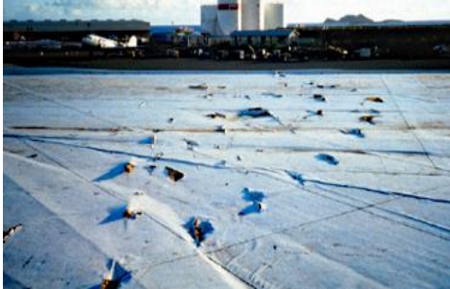
(a) Membrane damage (Smith 2017)
