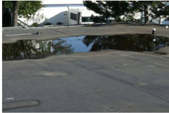
Figure 3-36. Water ponding areas (Roof Slope 2016)
