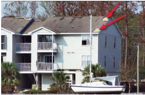
(a) Roof covering damage
