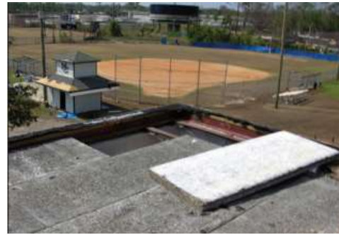
(b) Deck panel blow off at a roof corner
