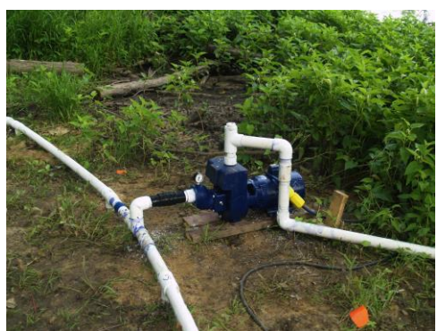
Pumps like this one are required to drain water from the fort site to allow excavation. Photo by Tori Hawley.
